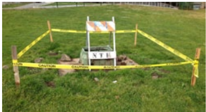
A complicated main water line break resulted in a large hole near the utility box outlet on the upper lawn
