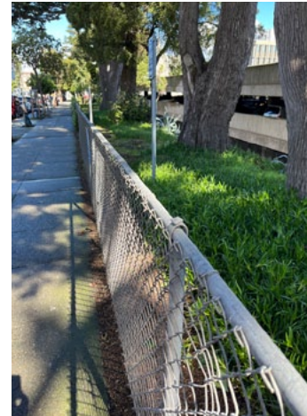
The CPMC campus perimeter on Castro is cut off from the neighborhood by unattractive chain link fencing.
